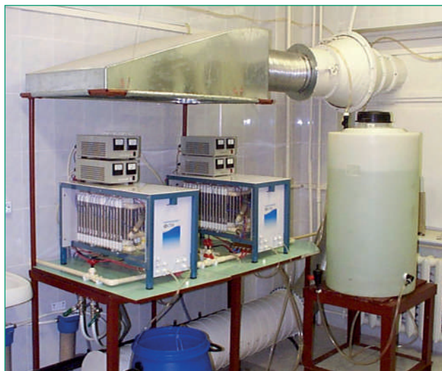
Fig. 6.3.7. STEL devices (NPO EKRAN) for the production of Anolyte ANK (500 l/h) in the «Anolyte» room Moscow City Hospital № 915, Moscow, 1999.
